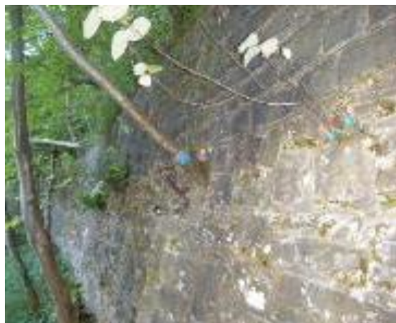
Trees on retaining walls marked with blue spray paint. There is evidence of trees having been removed along the wall by persons unknown and this could be attributed to the demarcation method employed.
